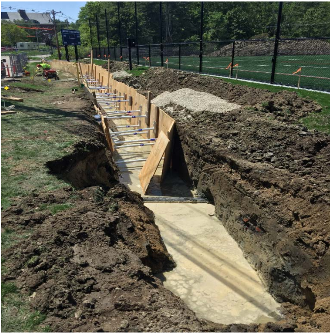
Fig 1: The trench that was flooded due to the water line break. Viewing south. (Approx. 1330 on Jun 3, 2019).
