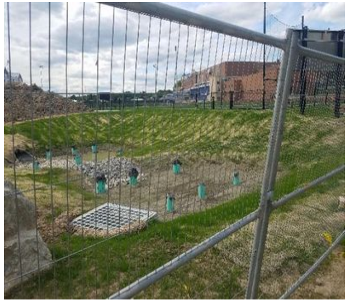
Fig 8: Rain garden. The water has drained and subsided. Viewing west. (Approx. 0630 on Jun 4, 2019).
