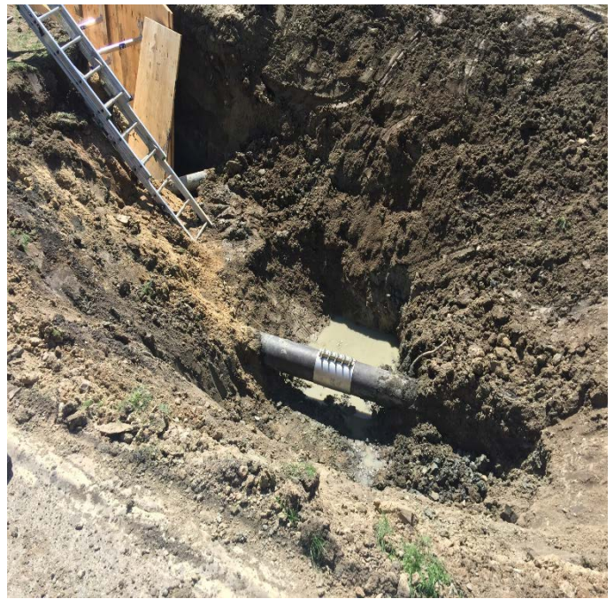
Fig 2: The water line repair patch. Viewing west. (Approx. 1330 on Jun 3, 2019).
