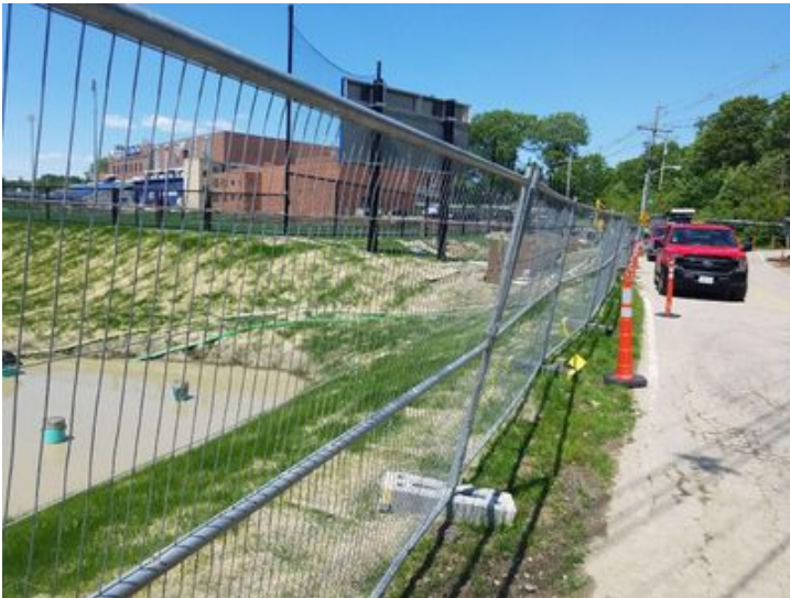
Fig 3: McCourt pumped the water out of the trench and discharged into the Rain garden along Colovos Rd. Viewing north. (Approx. 1330 on Jun 3, 2019).
