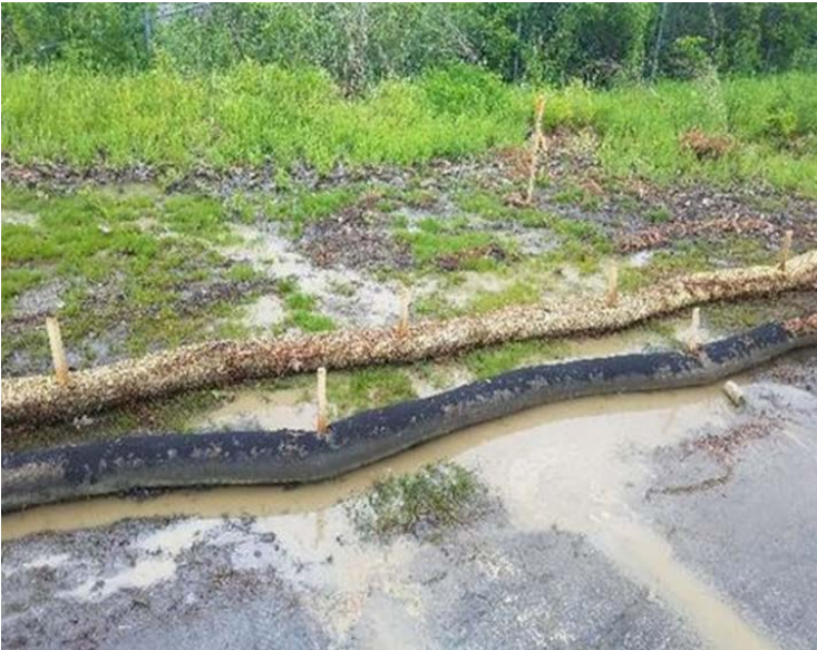
Fig 11: Low area in A lot where McCourt will install additional BMPs. Viewing east. (Jun 6, 2019).
